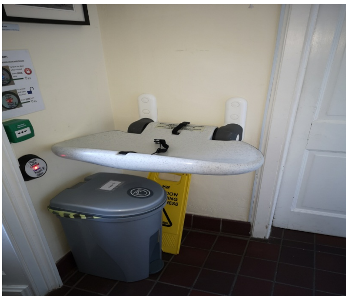
Baby changing facilities within the Accessible Toilet
