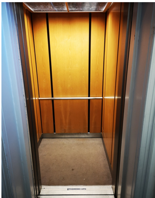
Interior of the lift
